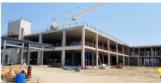
North West corner at the Emergency entrance and EMS ambulance bay steel structure
