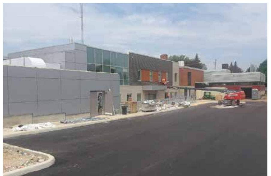
New two-storey addition housing ambulatory care department, day surgery, boardroom and offices.
